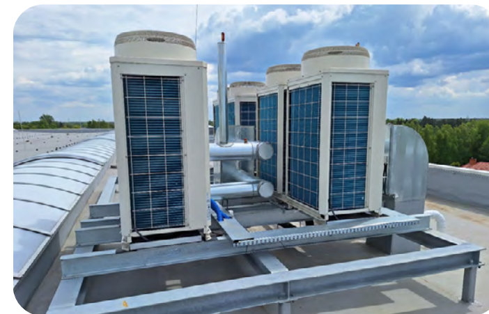
Heat Pumps Installed in the New Warehouse in Radzymin
